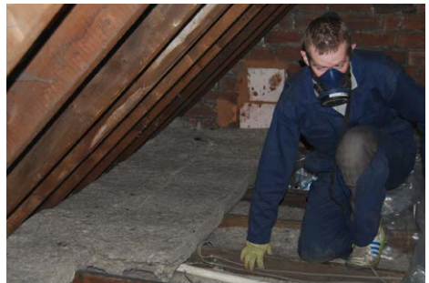
Sheep's wool insulation installed in a loft space which will help to reduce energy demand and improve thermal comfort.
